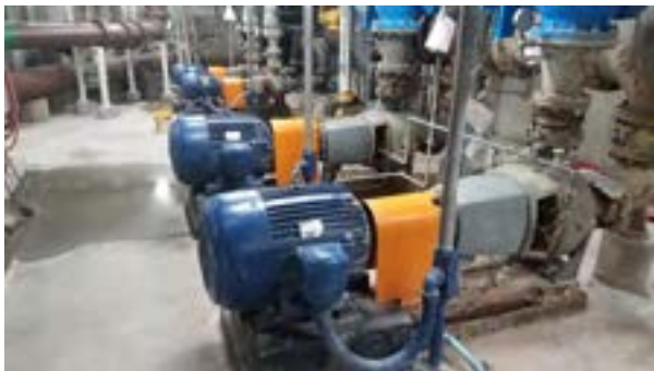
Pump motors in blue at one of the plant buildings
