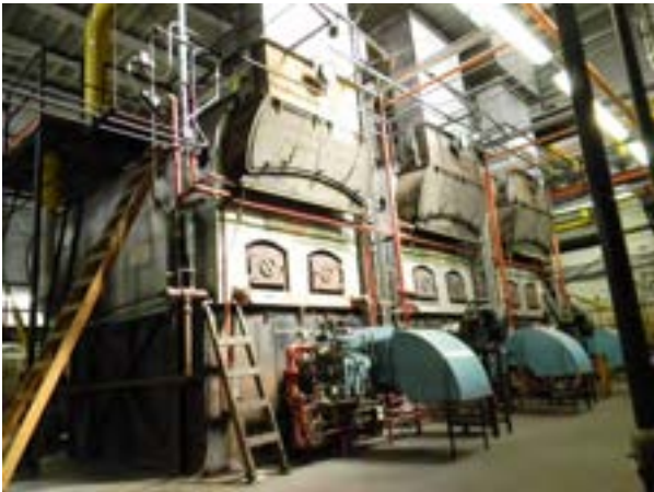
Heating boilers at pump station no. 6
