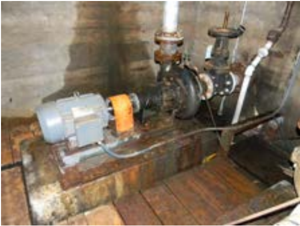
Sanitary lift station at
