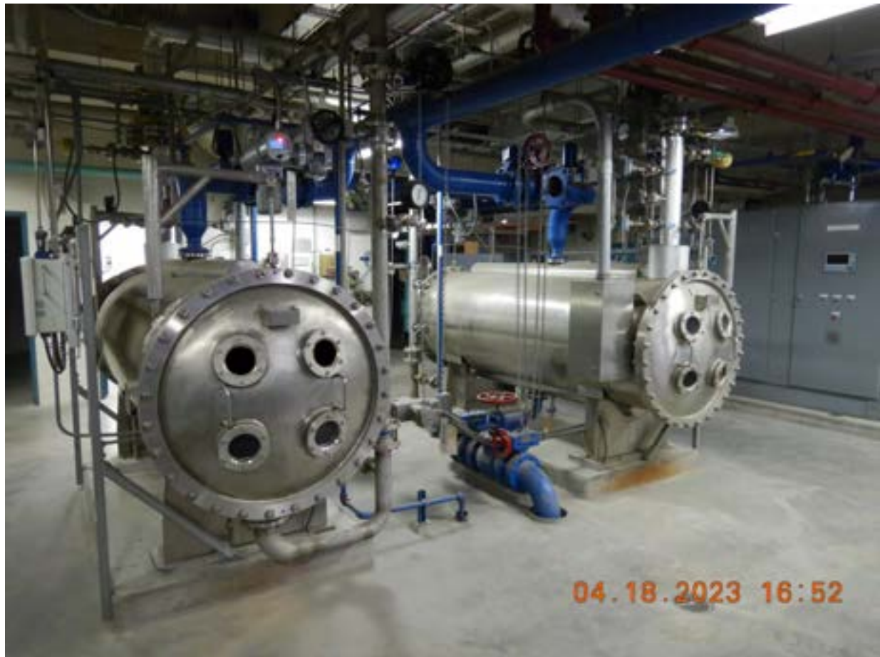
Figure 1: City of Fargo ozone generators
