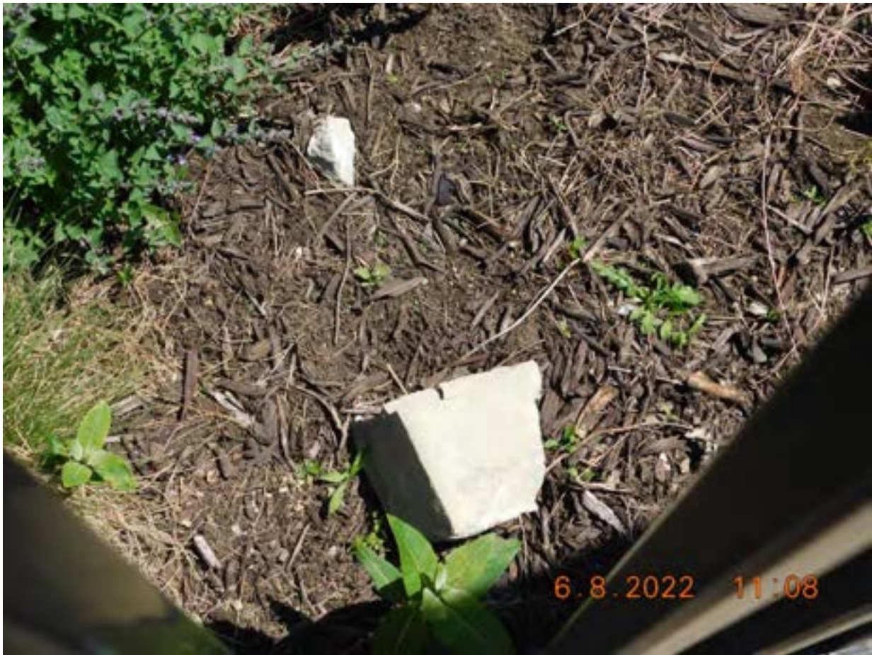
Observed fallen concrete at the base of the Washburn Tower
