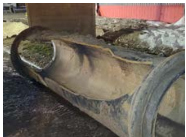
The cast iron pipe showing the missing portion of the pipe.
