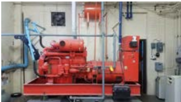
Obsolete emergency generator in one of the pump stations
