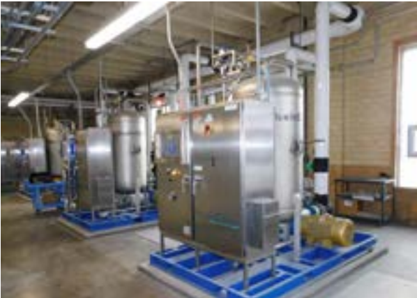
Recently installed CO2 equipment
