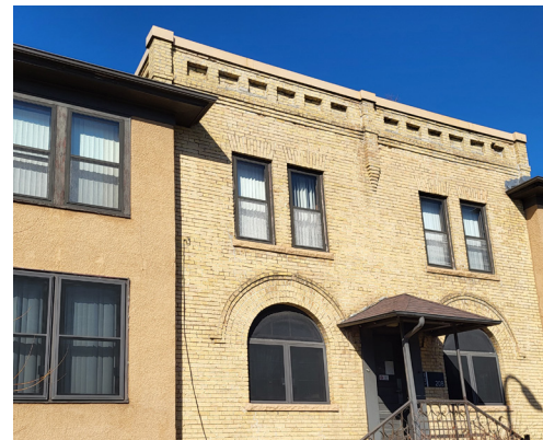
The storm windows at 206, 208, and 210 26th St E are pre-finished metal. Storm windows help retain heat inside the building.
